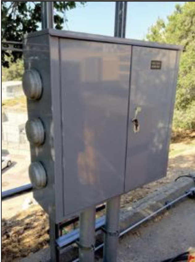
Figure 6: Cables to Mesa antenna farm and cable junction box next to building 329
