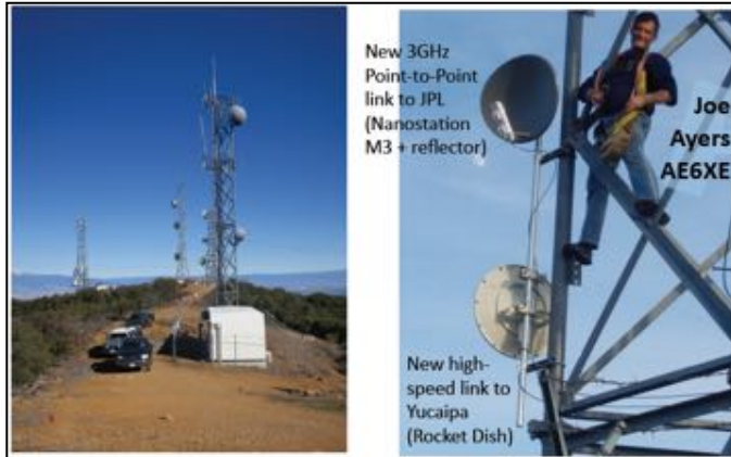
Figure 2: Installation of the JPLARC mesh node on Pleasants Peak, Orange County
